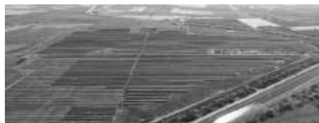
30 MW capacity solar power plant located in Raichur district of Karnataka state under group captive model
