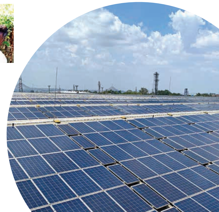
Roof top solar at Nashik plant
