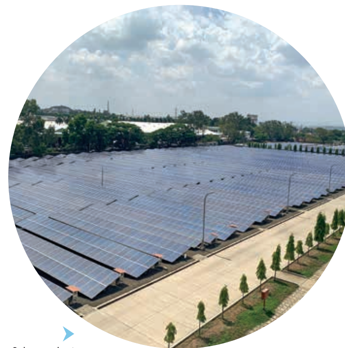
Solar panels at Nashik plant
